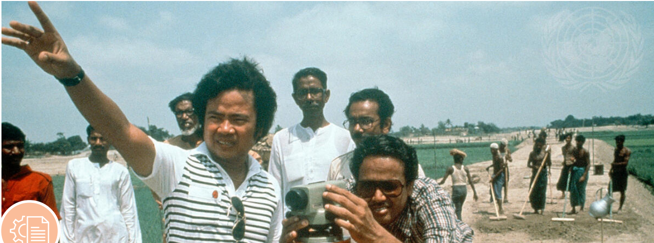
Filipino volunteers work on road construction in Bangladesh. [c.2001] (Source: UN Photo – International Year of Volunteers – 2001)
